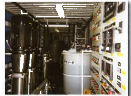
Containerized RO system
