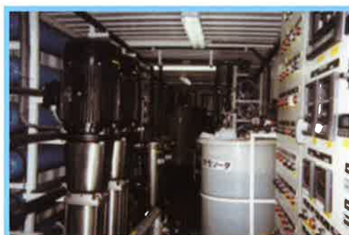
Containerized RO system
