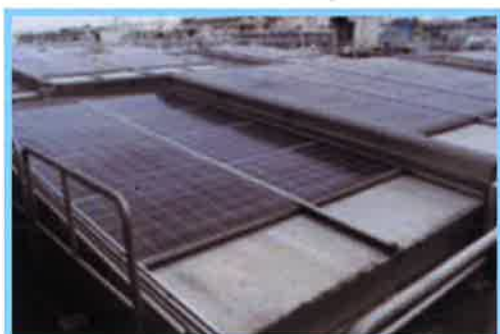
Solar powered system
