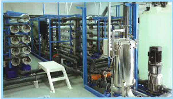
3,000,000 litres/day production capacity MBR-RO in Dubai, UAE
